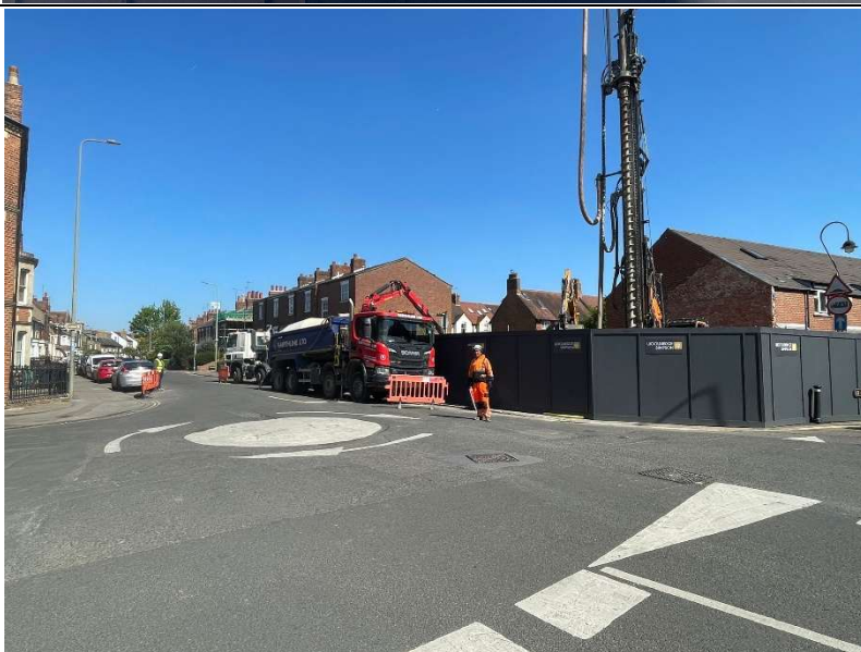
Piling operation in progress with Grab Lorry clearing excavated material, operatives marshalling the operation.
