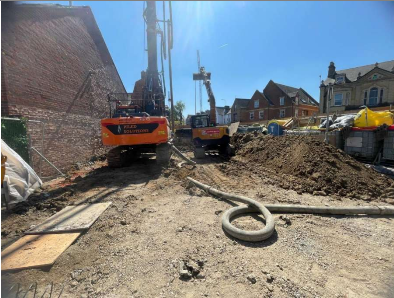
Piling in progress with standby digger clearing spoil as it arises to heaps.
