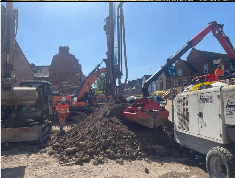
On site view with off site Grab Lorry clearing excavated material to create space for further piles.
