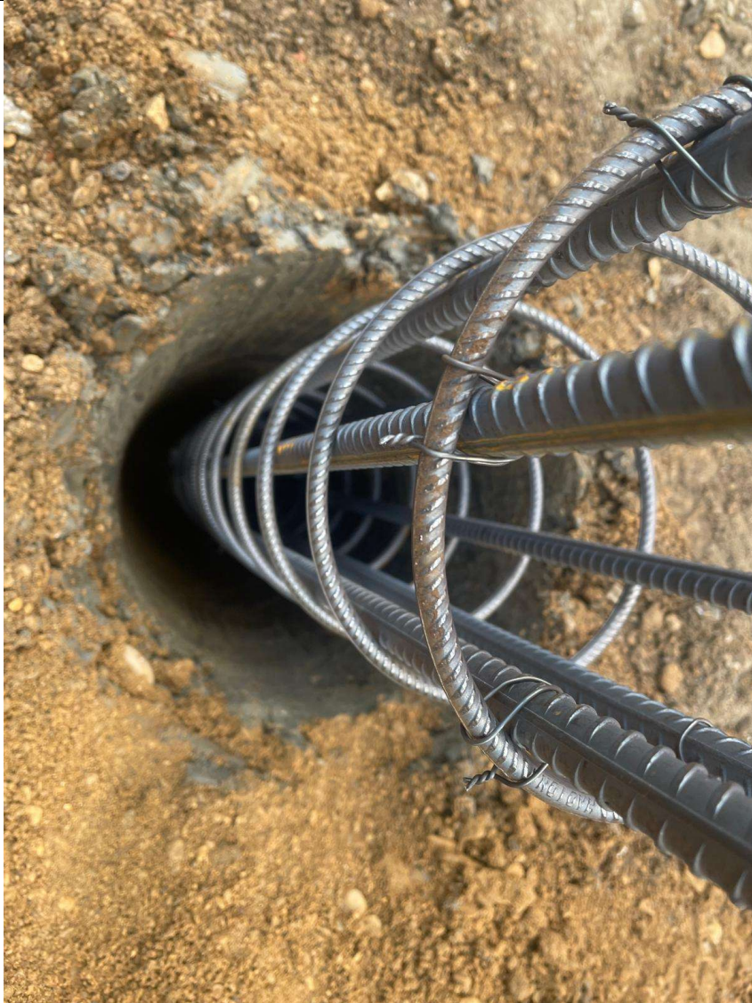
Typical Pile bored 9.00 metres down into Oxford Clay with reinforcing in place ready for concreting.
