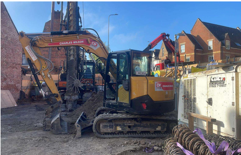
Site Area Piling rig operating with Digger moving excavated material into reach of Grab Lorry.
