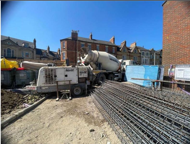
Site area with Reinforcing Cages and Concrete Pump receiving Concrete from on road delivery.
